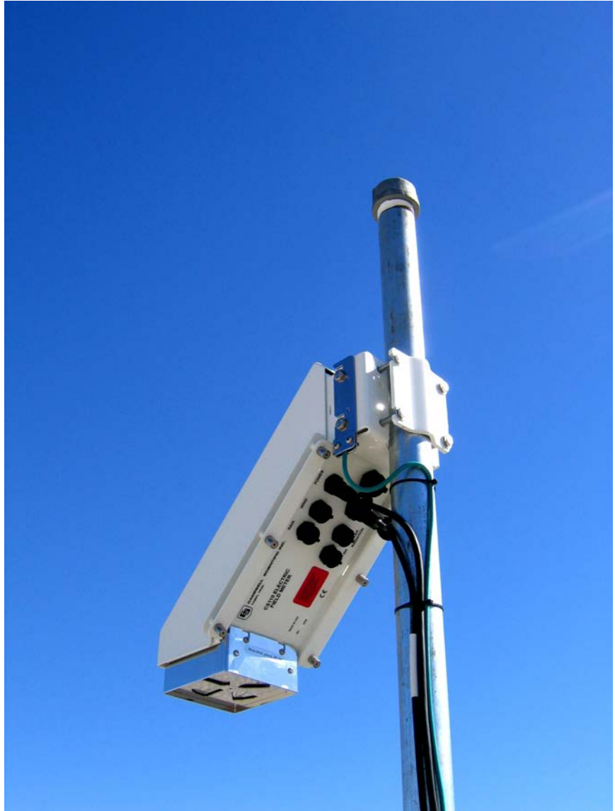
FIGURE G-2. CS110 on CM10 Tripod Mast
