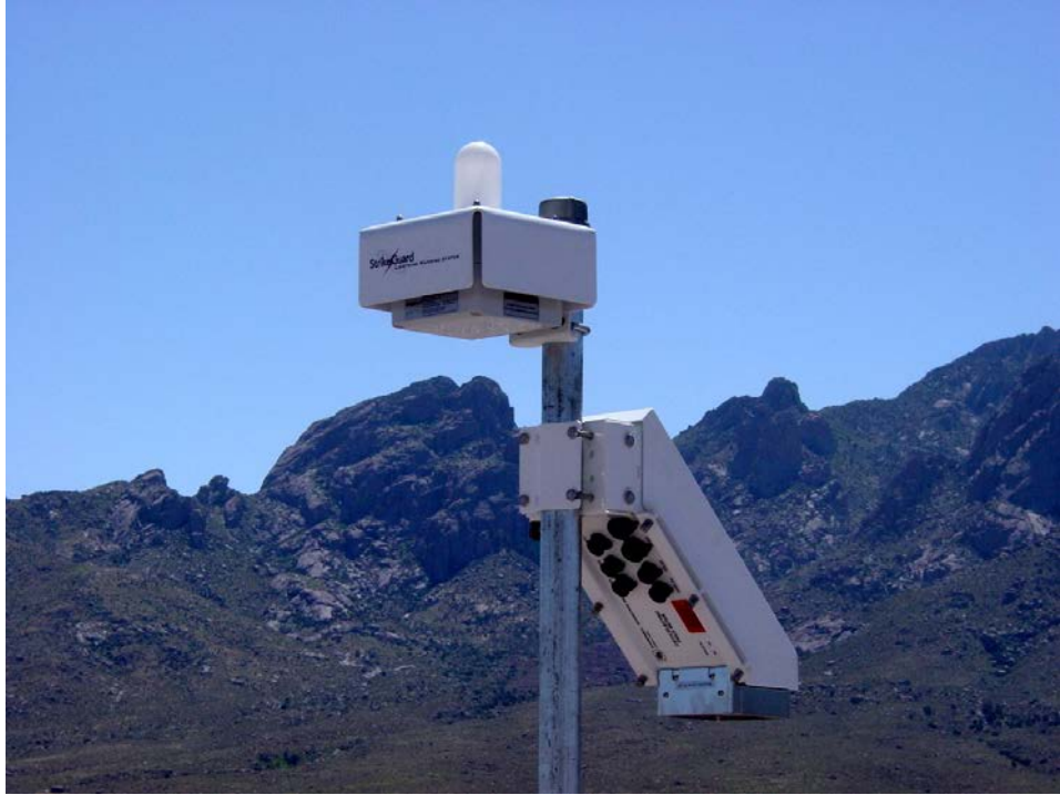
FIGURE H-2. CS110 and StrikeGuard on tripod mast
