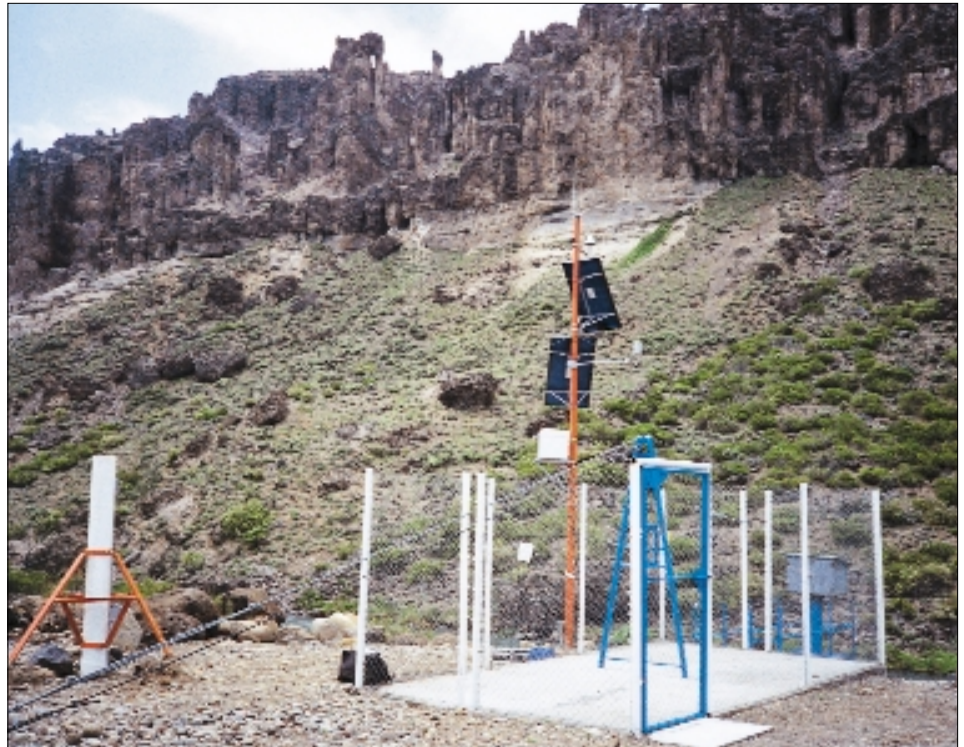
The Inmarsat-C satellite system provides telecommunications for remote Argentine stations.
