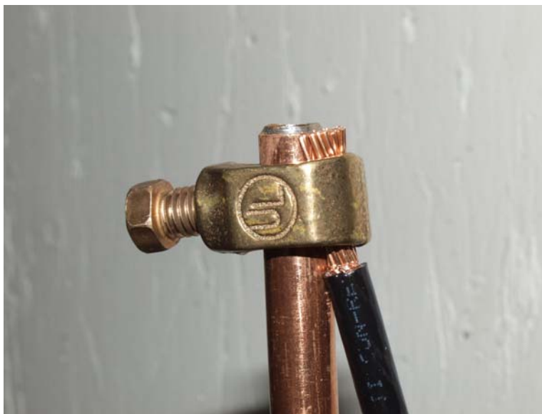
FIGURE 5-9. Ground Rod and Clamp
