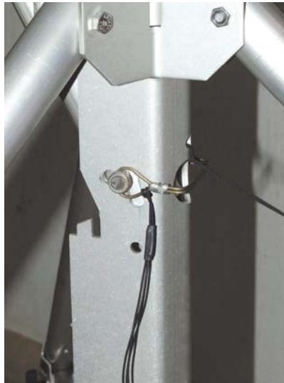
FIGURE 5-3. Mast Attachment to Tripod Base
