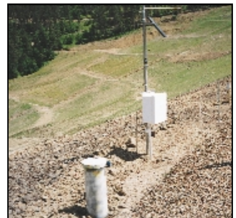
Wireless telemetry, in this case cell phones, simplifies data retrieval from remote areas.
