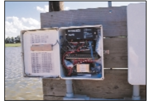
Though pond-condition data can be viewed and controlled via a personal computer, special display-equipped enclosures (shown open above) also make data visible on-site.
