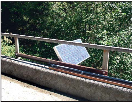
The system's solar panel was mounted off the side of a bridge spanning the Cedar River to avoid shading from the surrounding forest.
