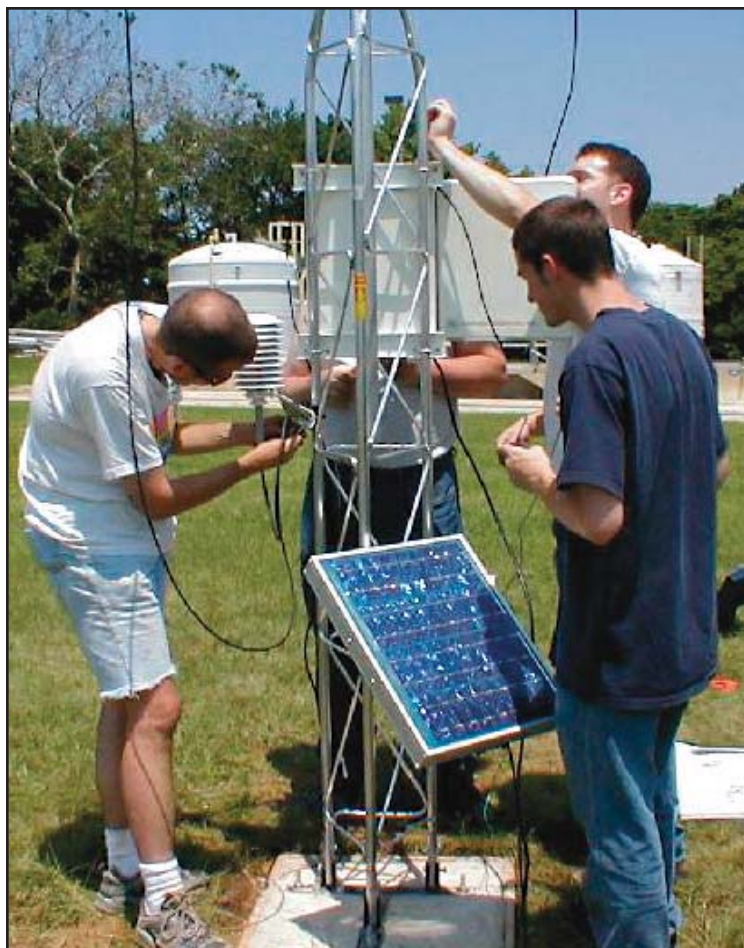
Installing a new DEOS station increases the area covered by the network, and allows graduate students at the University of Delaware to gain experience working with meteorological equipment in the field.
