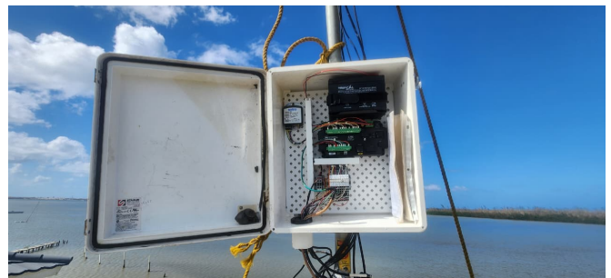
Inside the weather station enclosure
