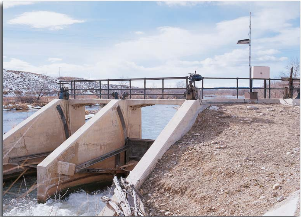
Our systems automate water management by measuring water level, adjusting gate height, and recording information—all unattended—every day, every night, all year long.
