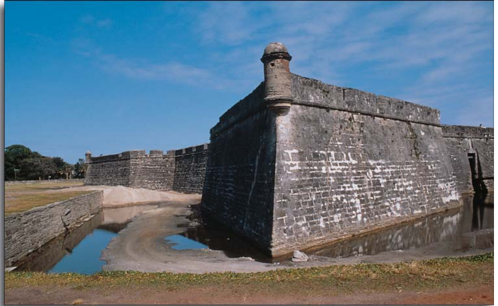
A preservation project at Castillo de San Marcos, St. Augustine, FL involves monitoring cracks in three dimensions, the tilt of the large segments between the major cracks, change of soil moisture within the bastion, and weather conditions at the site.
