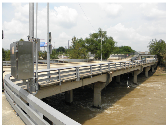
High water from Hurricane Harvey
