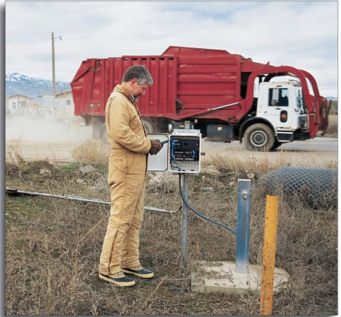
Our dataloggers are typically interrogated via telecommunications from an office, but you can also access the data on-site.
