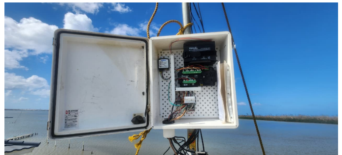
Inside the weather station enclosure
