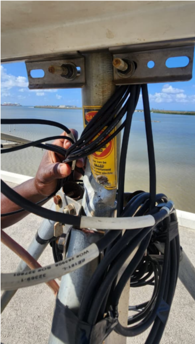
The bent center mast after the station survived the hurricane
