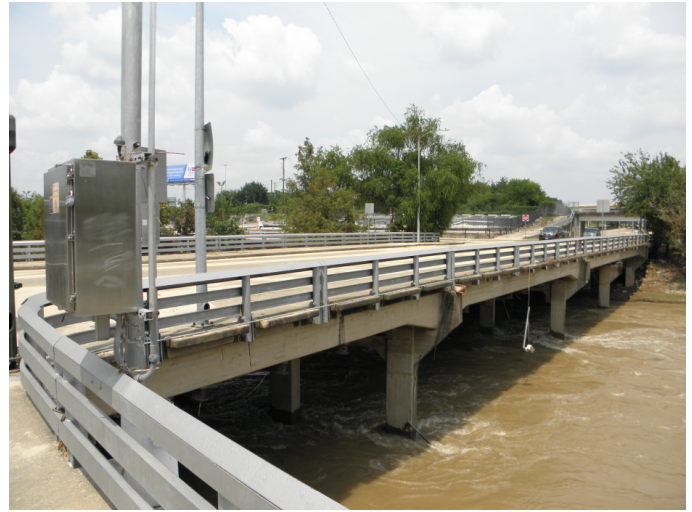
High water from Hurricane Harvey
