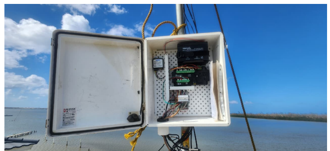
Inside the weather station enclosure
