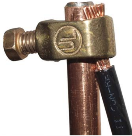
Figure 5-11. Ground Rod and Clamp
