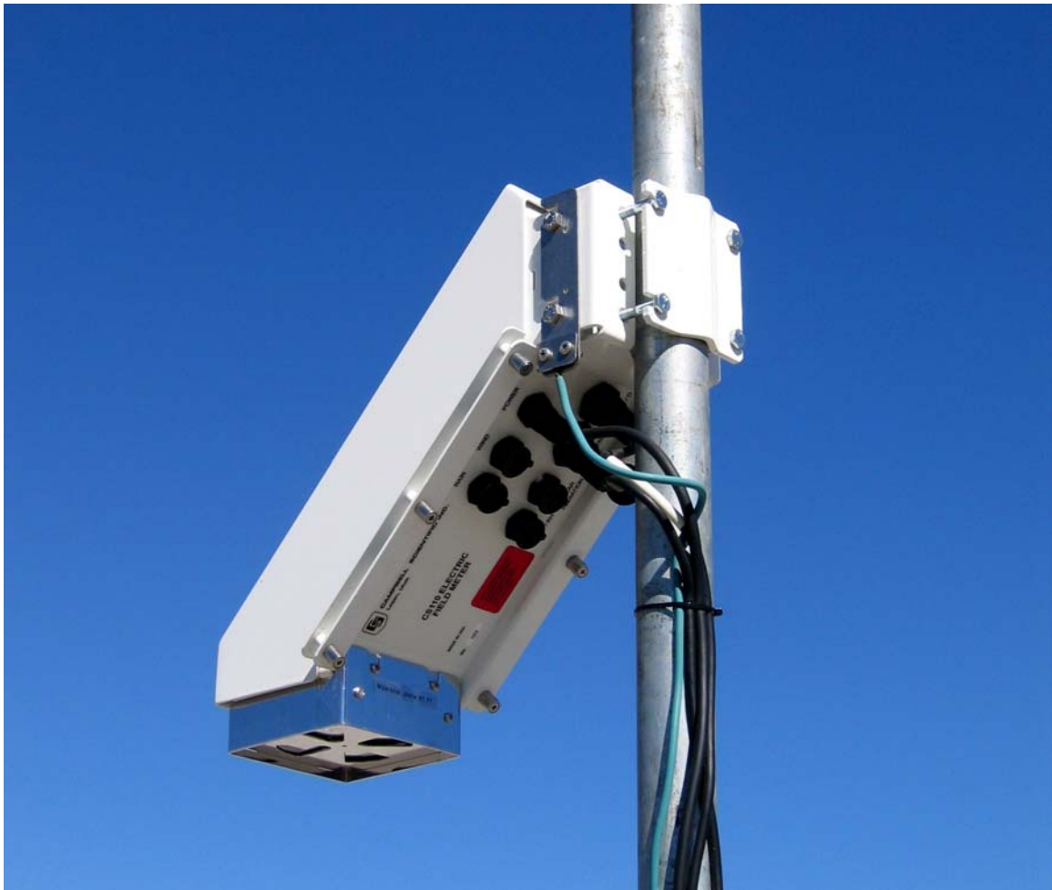
FIGURE H-3. Grounding the CS110 Grounding Strap
