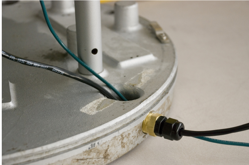
FIGURE 3.3-1. Solar panel cable and grounding wire routed through compression fitting of rain gauge base.
