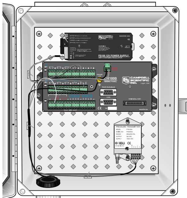
FIGURE 3.2-1. Routing and Wiring Sensor Leads to the Datalogger
