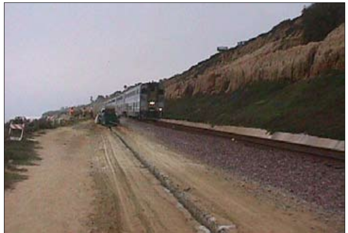
TDR cables are buried parallel to the track in a layer of concrete.
