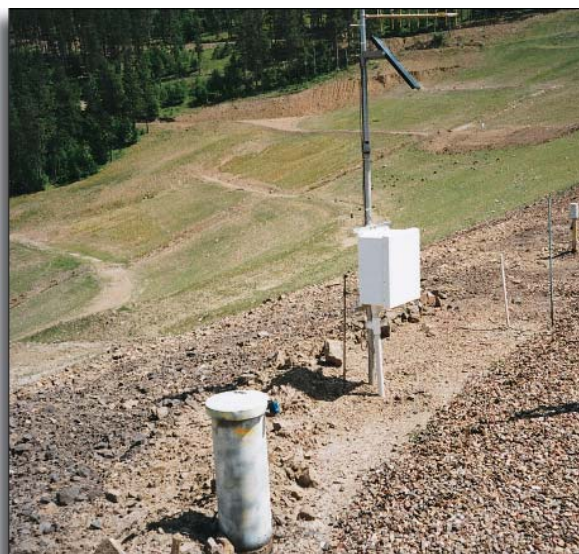
A variety of methods are available for monitoring the performance of acid rock drainage caps.
