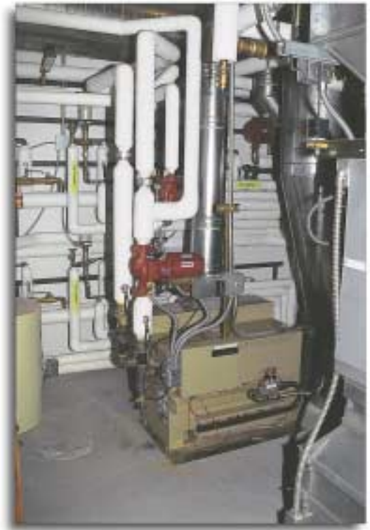
Our systems monitor and control pumps, fans, motors and many other devices. Proportional control of dampers or valves is also possible.
