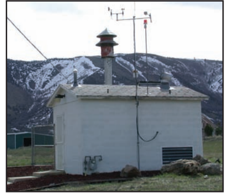
A system monitors water and meteorological parameters at a pump control site for the Mantua, UT, water system
