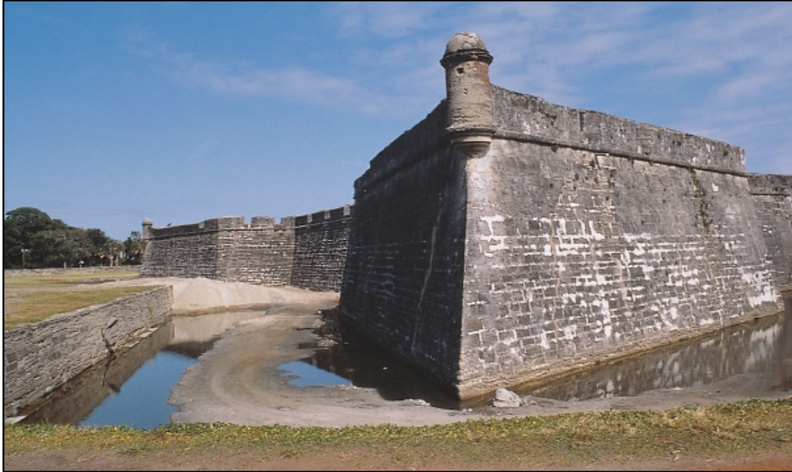
Castillo de San Marcos National Monument, St. Augustine, Florida. Taken in 1995, this view looks across the moat toward the southwest bastion, where several major cracks are visible.
