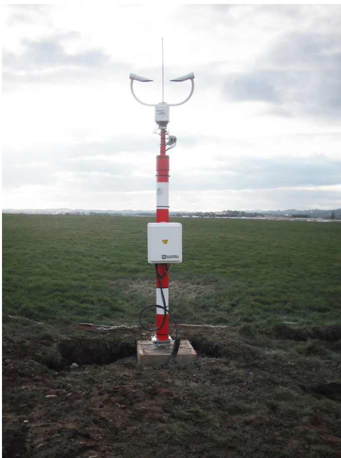
CS120A Visibility & CS140 Background Luminance Sensors mounted on a frangible mast
