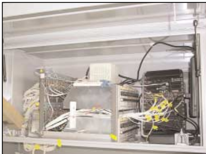
(Top) An enclosure housing a CR9000 system is bolted to a floor beam underneath the Williamsburg Bridge in New York City.
