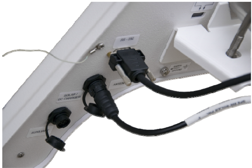
FIGURE 2-18. The Cables Connected to Weather Station
