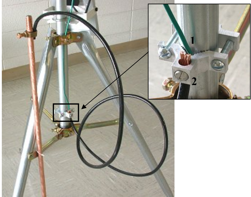
FIGURE 2-13. The right close up is the 14 AWG wire and the #4 cable attached to the tripod coupling.
