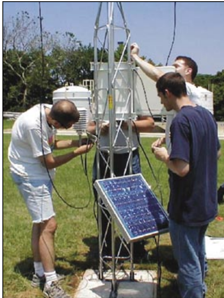
Installing a new DEOS station increases the area covered by the network, and allows graduate students at the University of Delaware to gain experience working with meteorological equipment in the field.
