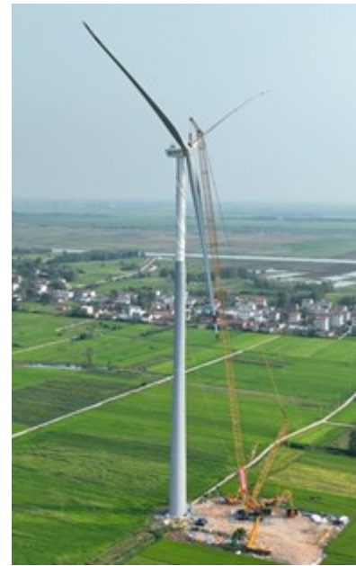
Goldwind recently installed the world's tallest onshore wind turbines in China, featuring a steel-concrete hybrid tower standing at a height of 185 m (607 ft). (Photo courtesy of Goldwind)
