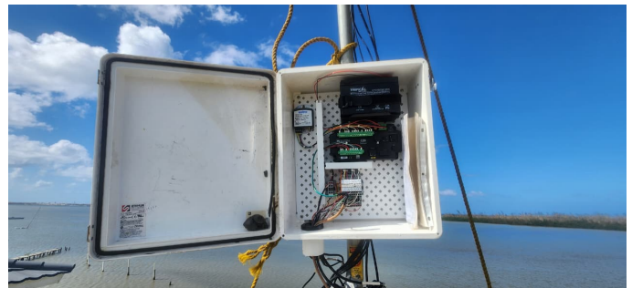
Inside the weather station enclosure
