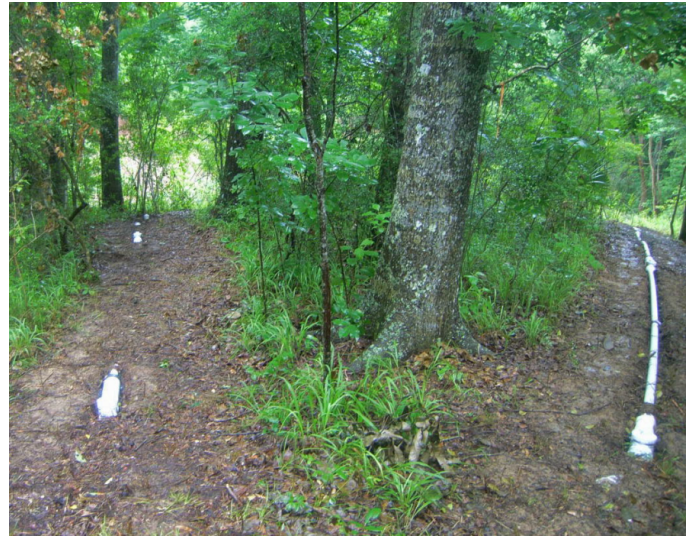
Two of the three arrays of telescoping PVC running from the data logger to the edge of the sinkhole
