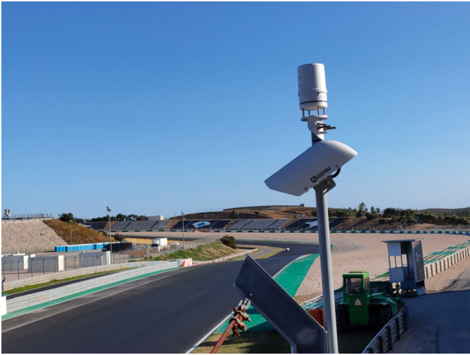
The installation of the digital weather sensor and non-invasive surface temperature sensor
