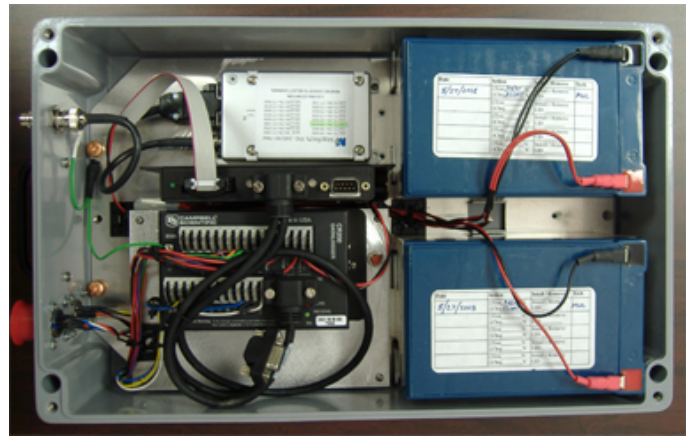
Data logger, communication gear, and batteries in enclosure
