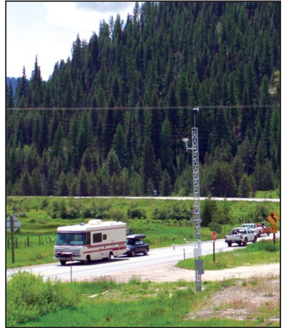
Roadside Environmental Sensor Stations (like the one shown above) monitor real-time road conditions and telemeter data to a central DOT office.
