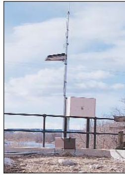
Up to 254 sites can be interrogated over a UHF or VHF frequency.
