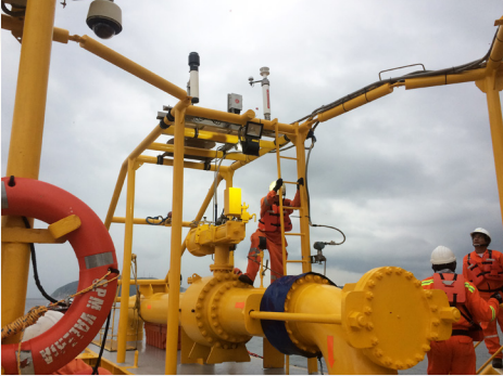
Solar-powered WEATHERPAK® on offshore buoy in Colombia
