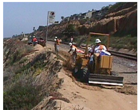
Campbell TDR system monitors slope stability ( www.campbellsci.com/slope-monitor )
